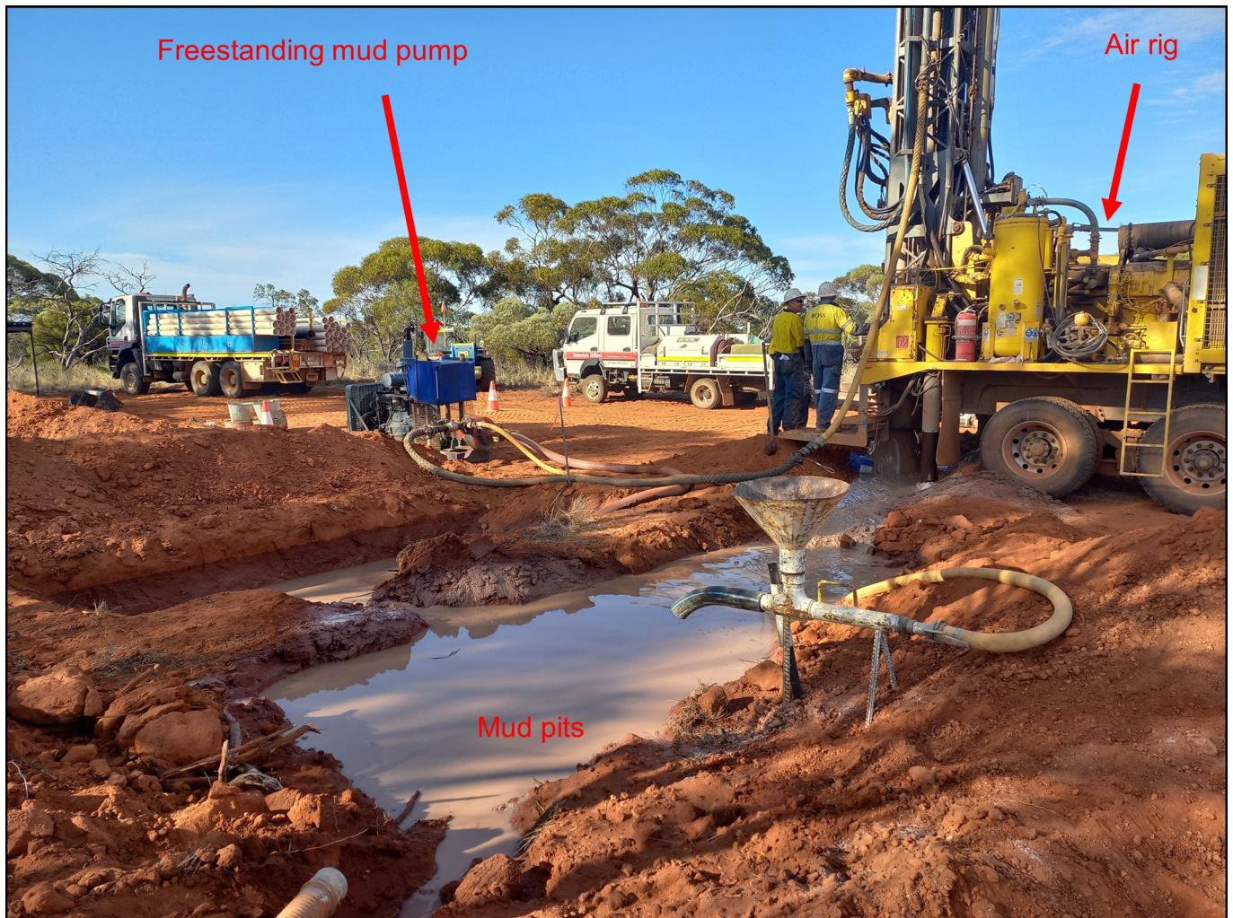
Figure 1: Photo of water boring drill rig at Hector. Pits were established to mix the “muds” required to stabilise holes and to ensure no discharge of water and material to the environment.
