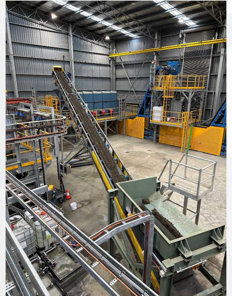
Concentrate Dryer and Magnetic Separator
