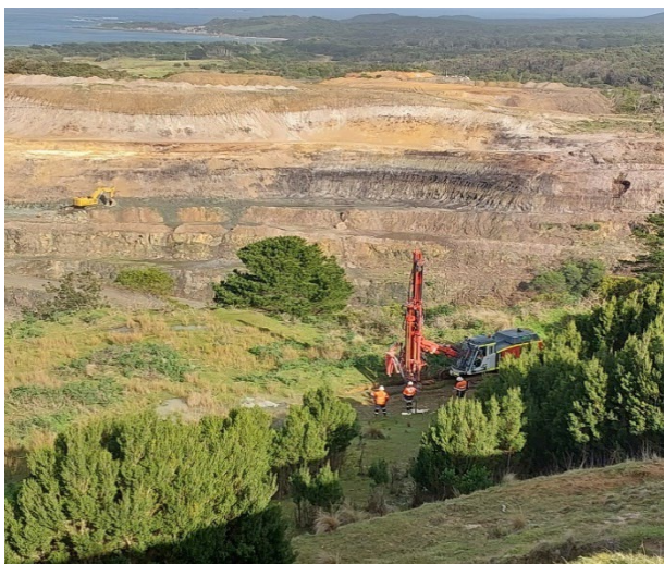
Figure 4 – Commencement of drilling on north cut back of the Dolphin open cut
