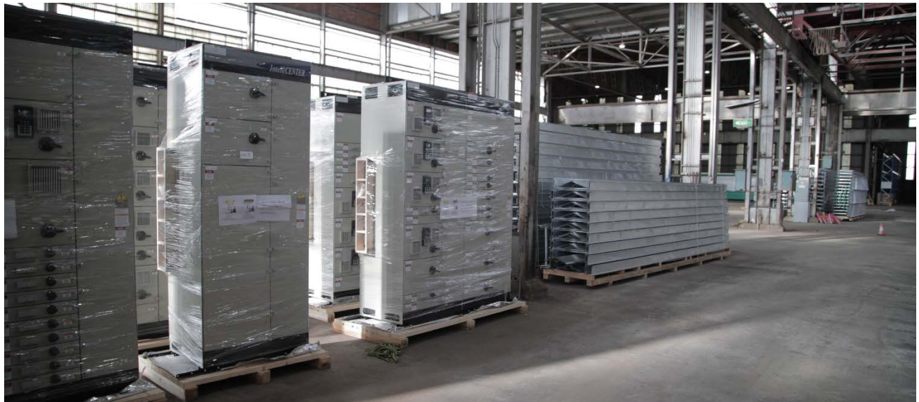
Figure: Motor Control Centers (MCC) & Cable Trays On-Site
