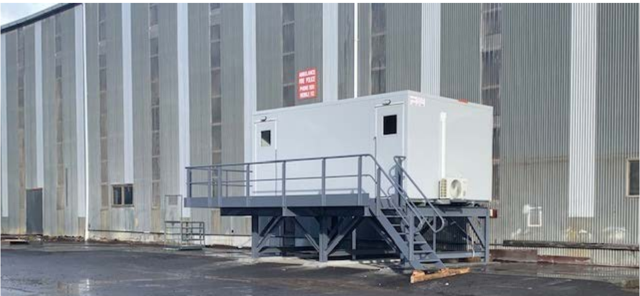
Figure: Hydromet and Reduction Area Switchrooms Installation Complete
