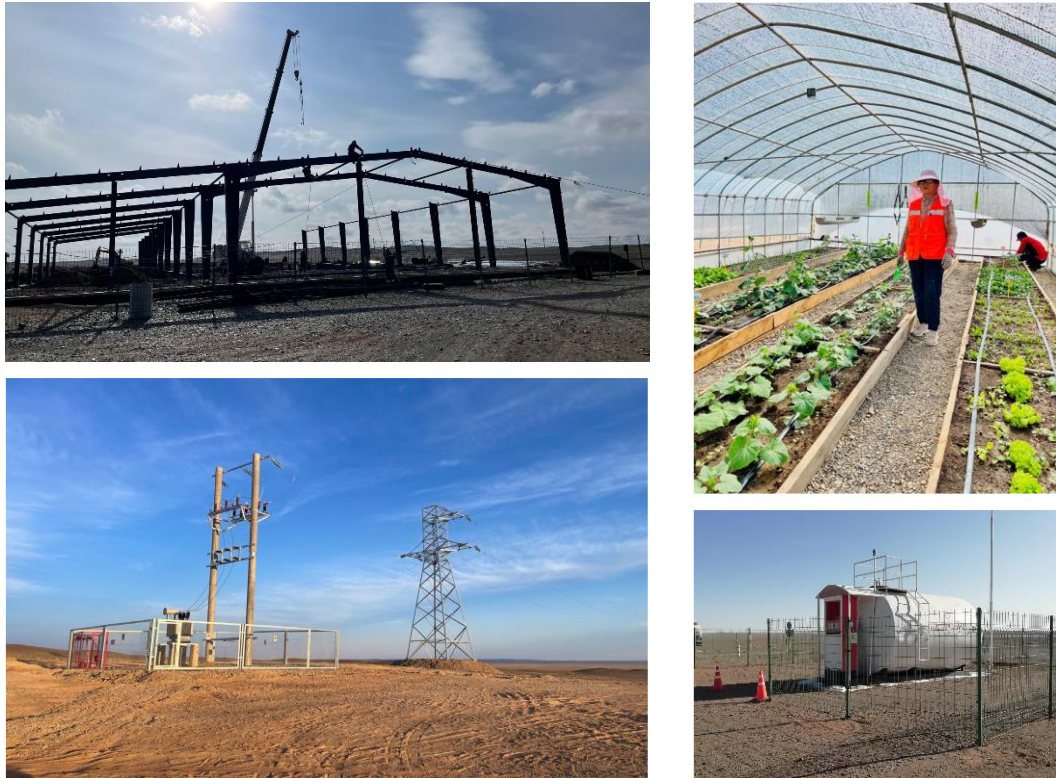
Figure 2. Clockwise from Top Left – Core Processing Facility, Greenhouse, Drinking Water Filtration System, 35kV Grid Power Supply
