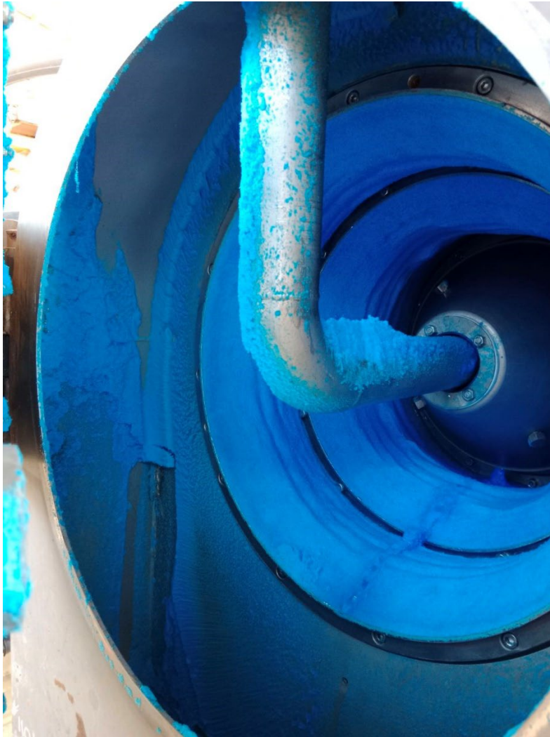
Figure 2: Picture of the centrifuge loaded with copper sulphate crystal produced at the Cloncurry Project Copper Sulphate Plant
