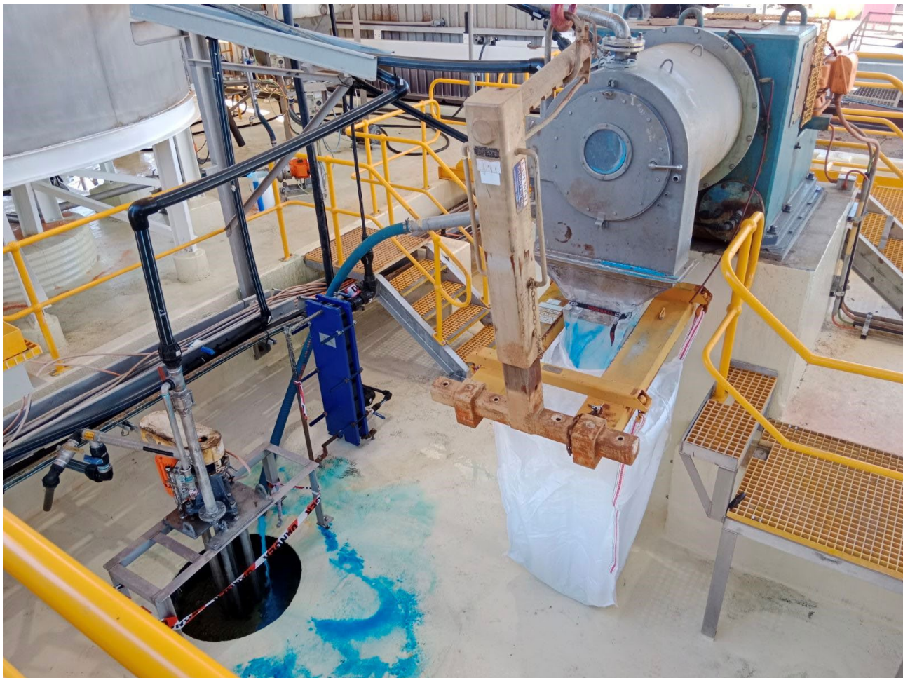
Figure 1: Copper sulphate crystal loaded into a Bulka bag from the plant centrifuge at the Cloncurry Project Copper Sulphate Plant
