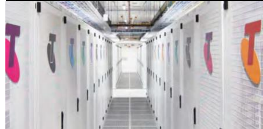
TELSTRA DATA CENTRE, CLAYTON VIC
