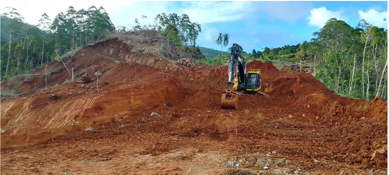
Photo 1. Haul road construction on schedule, heading up to the first ore blocks
