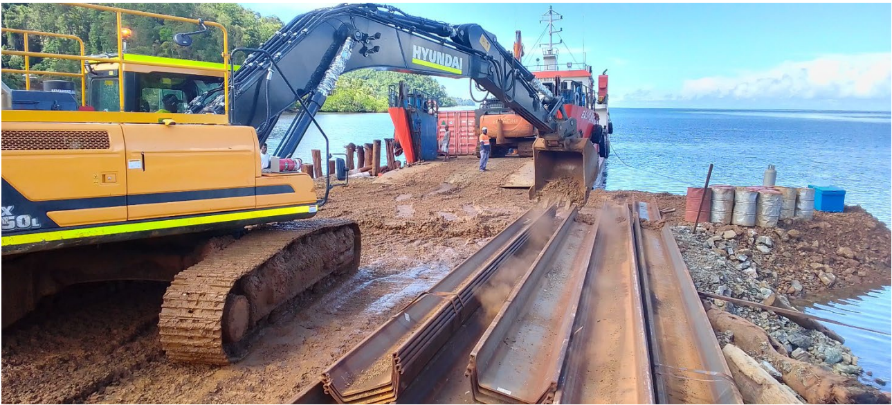
Photo 3. Sheet piles to be used in construction of the Wharf arriving at Kolosori
