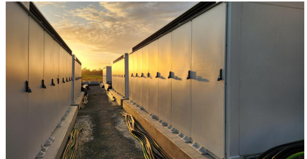
Figure 2: Tesla Megapacks at BBP Project
