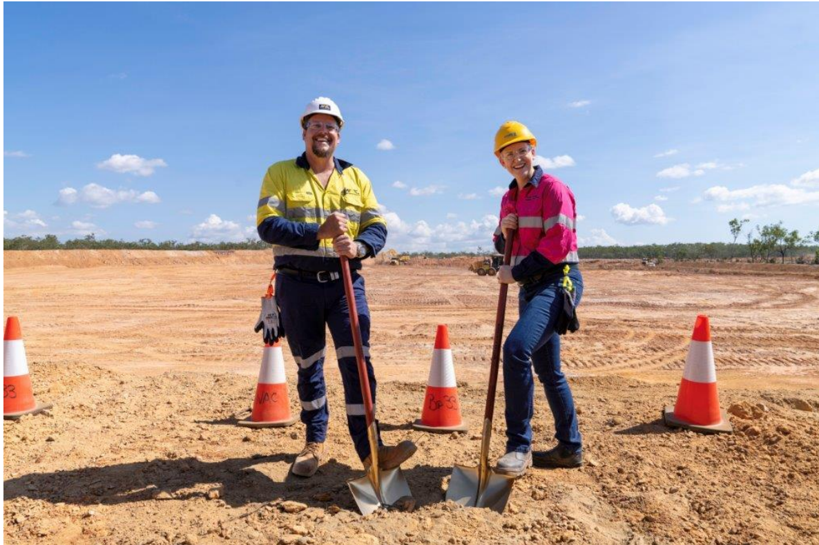
Northern Territory Minister for Mining and Industry, the Honourable Nicole Manison, attended the official sod-turning event at BP33 on 17 August 2023 – along with Northern Territory contractors Northern Australia Civil and members of the Core Lithium leadership team.
