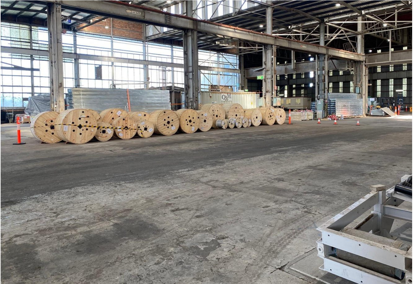
Figure: 30km of Power and Instrumentation Cable
