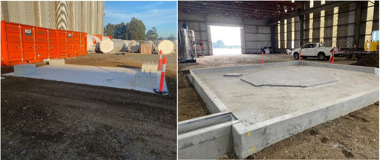
Figure: SCM Silo (left) and Magnesite Silo Mixing Tank (right)
