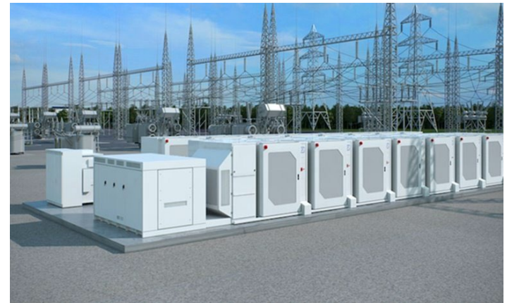
Full BESS System
