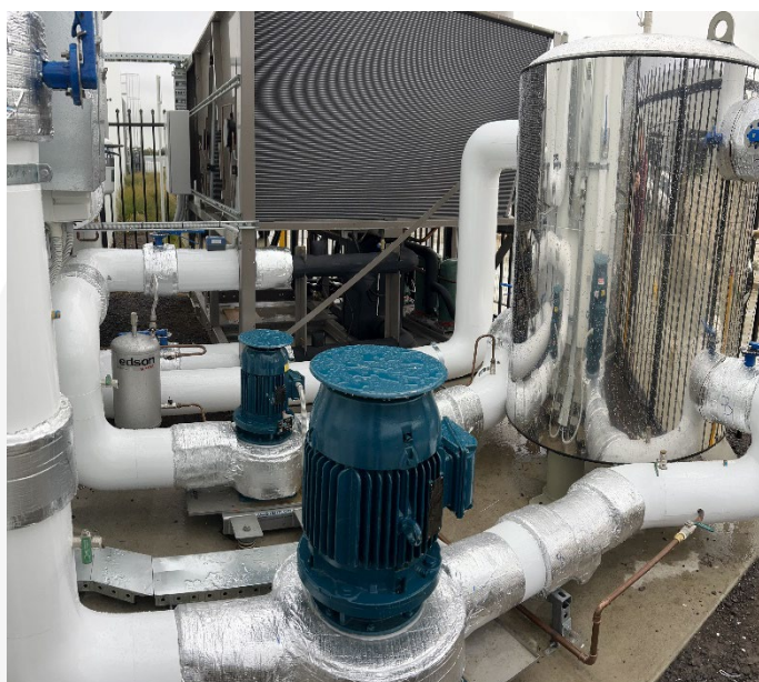
2. The external chiller
