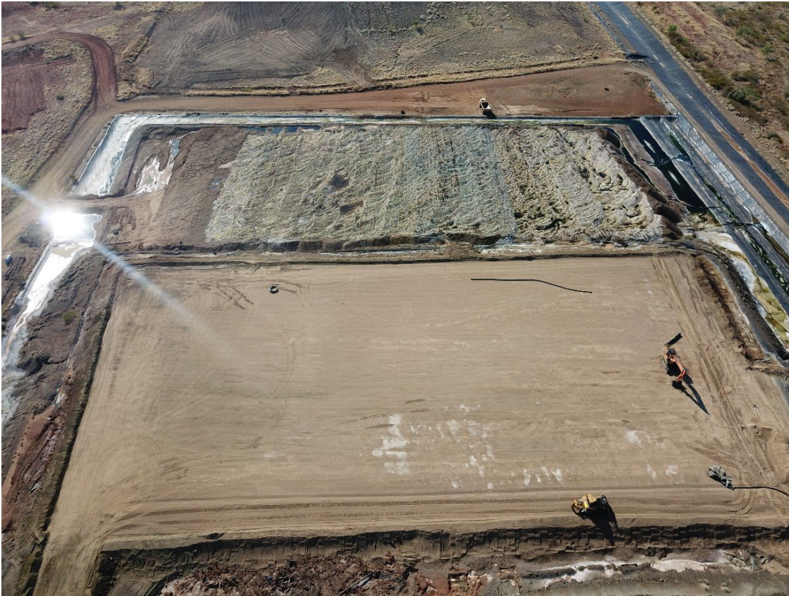
Figure 2. Great Australia Heap Leach Pad 6, stacked and under leach. Pad 5 prepared for receiving material in the foreground.
