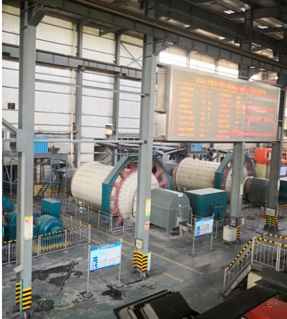
Prominer 650Ktpa Grinding Circuit
