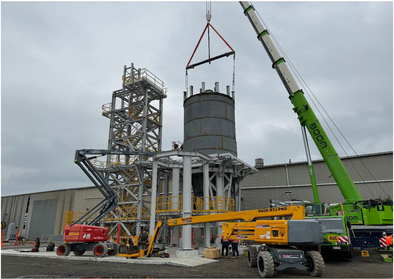
Figure: Spray Roaster reactor vessel installed in final position
