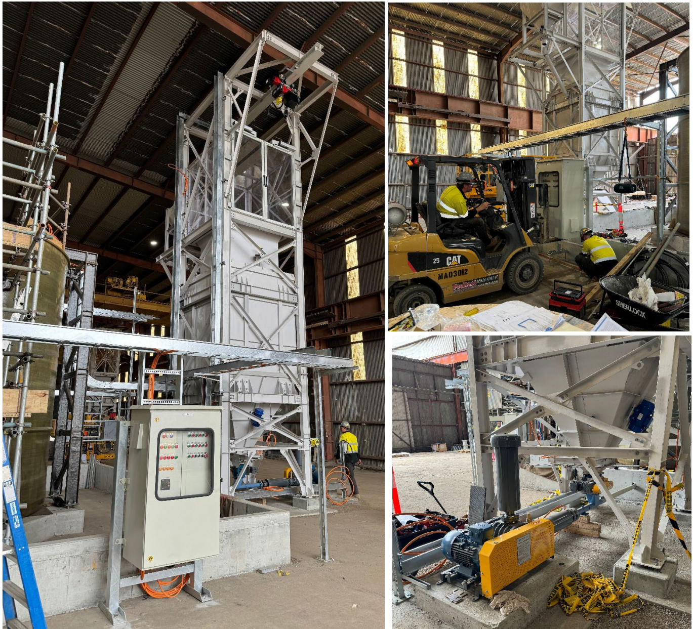
Figure: Magnesite Hopper & Bag Breaker unit E&I and Mechanical equipment installation completed.
