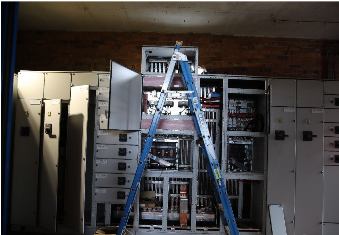
Figure: New Main Switchboard (MSB) installed and powered.
