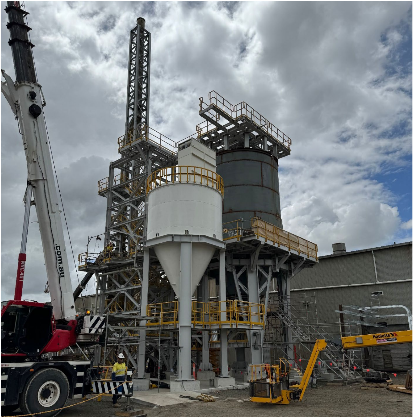
Figure: Spray Roaster's reactor vessel & oxide bin installed along with structural steelwork erection complete.
