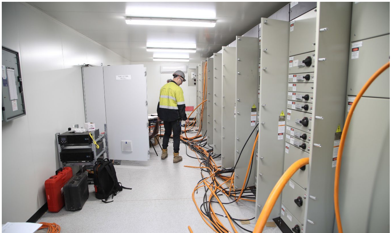
Figure: Electrical and instrumentation cable installation in cable trays & local junction boxes
