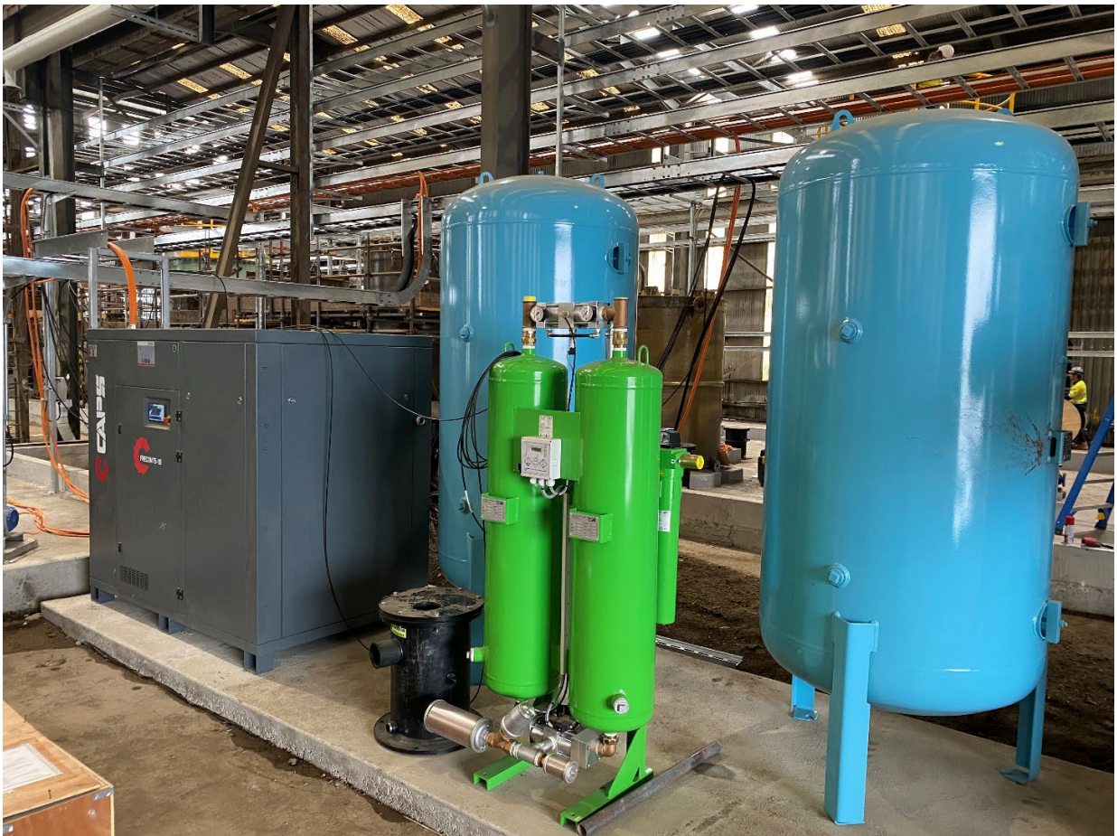
Figure: Filter area FRP tanks and air compressors installed
