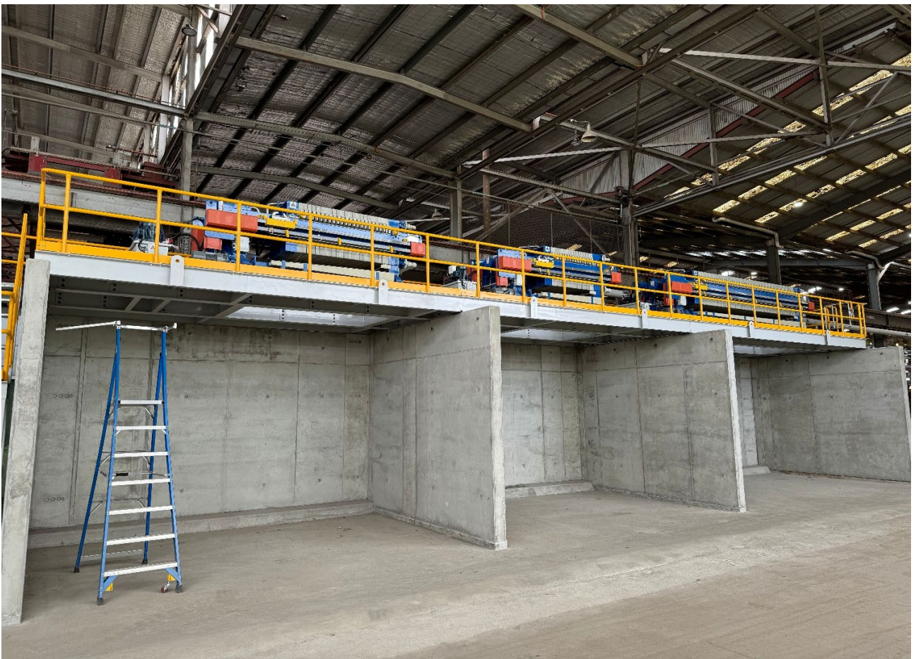
Figure: Filter Presses installed over Filter bunkers and all major mechanical equipment
