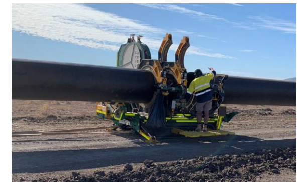
Polyethylene waste recycling program during installation of the rising main pipeline, Rookwood Farms, central Queensland, July 2023.
