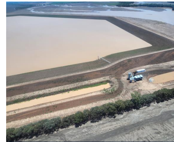
Pumps transferring water into the newly constructed water storages, Baamba Plains, February 2024.
