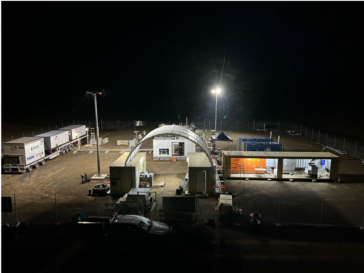
Figure 1: Completed CNG Facility with virtual pipeline trailer parked at the filling post, in preparation for commissioning
