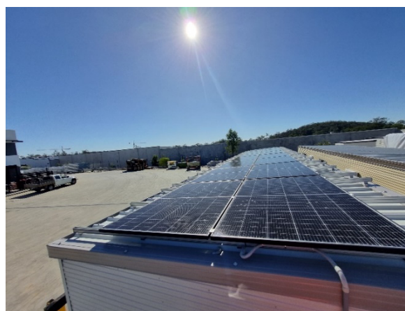
Figure 4: Solar Cells on accommodation dongas.
