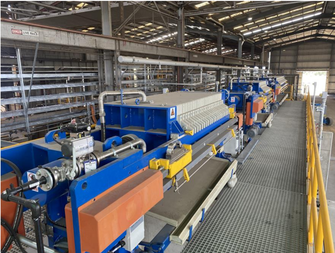
Figure: Filtration area complete with all piping, hydraulics and electrics installed
