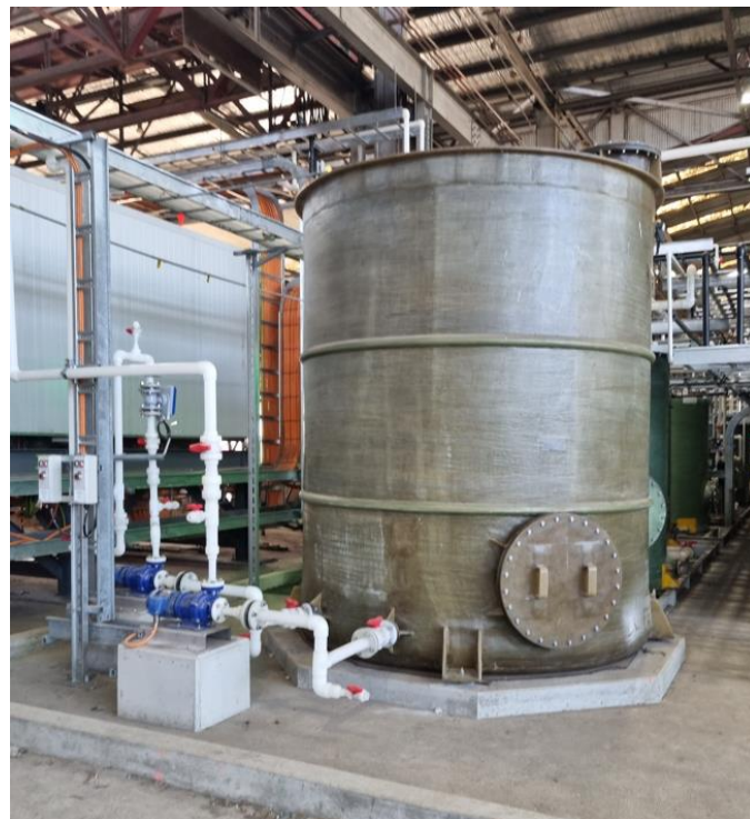
Figure: Magnesium holding tank complete
