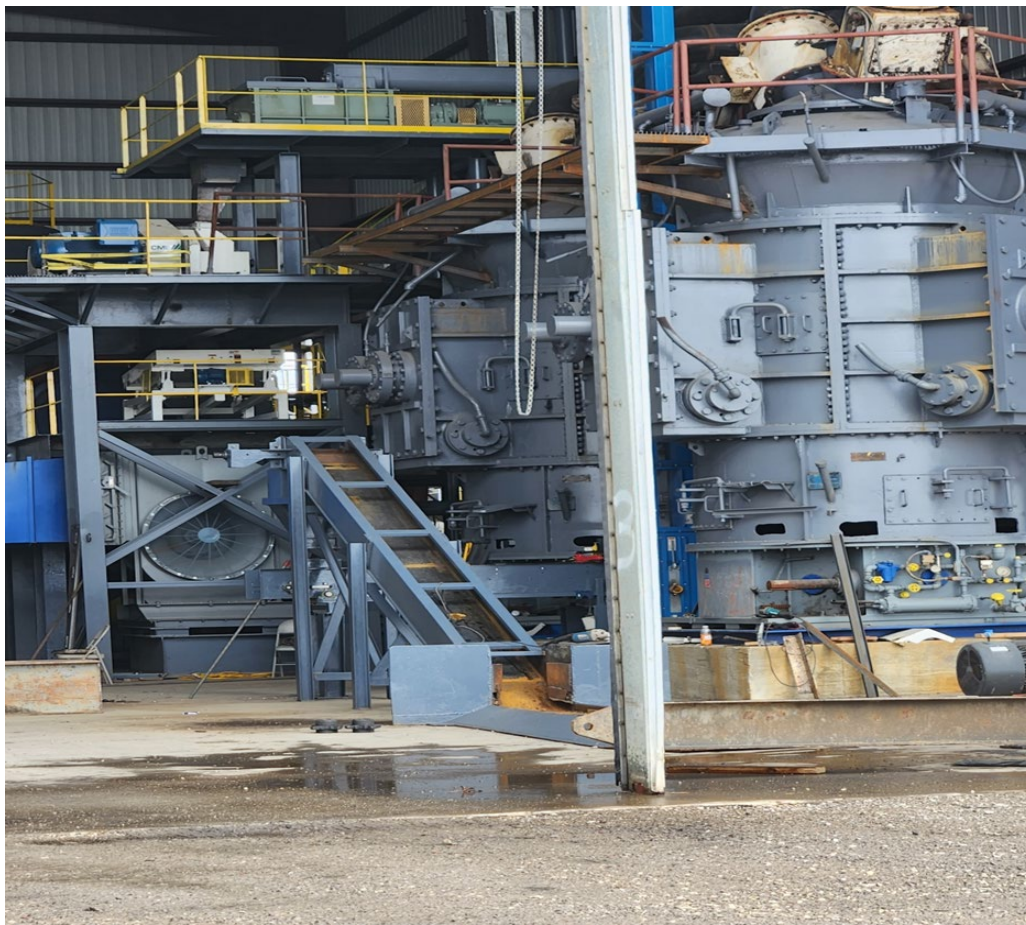
Image 1: Activated Carbon pellet plant close to completion ahead of first production run
