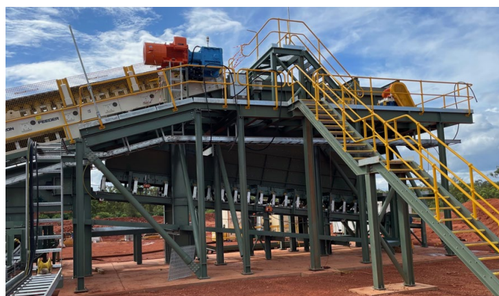
Apron and Wobbler Feeder Station
