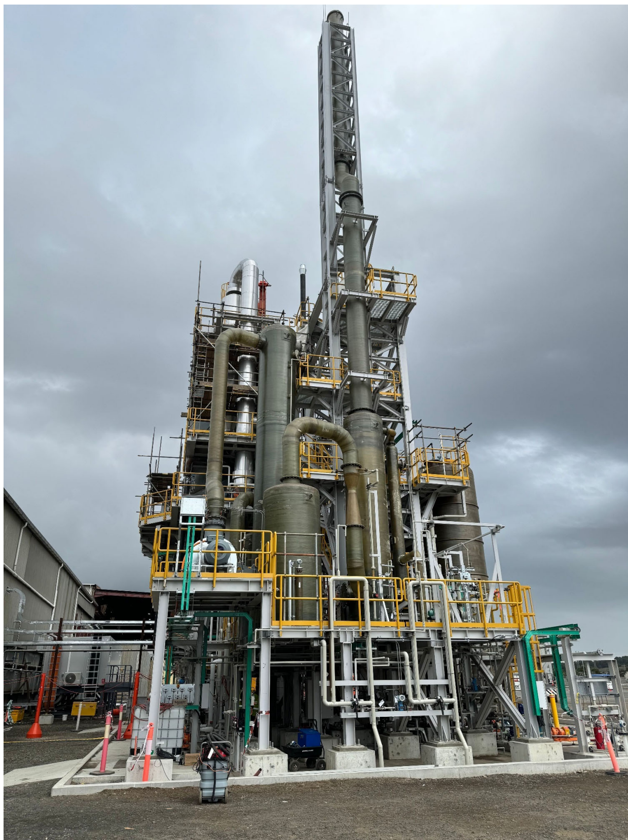
Figure: Spray Roaster's equipment installed and ready for final commissioning
