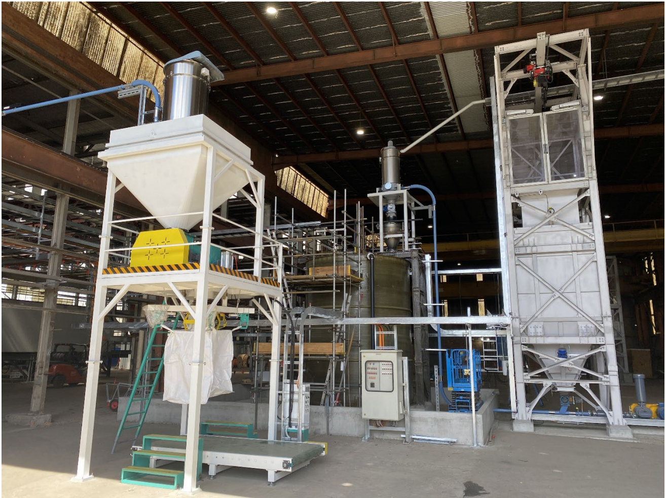
Figure: Magnesium Bagging Plant
