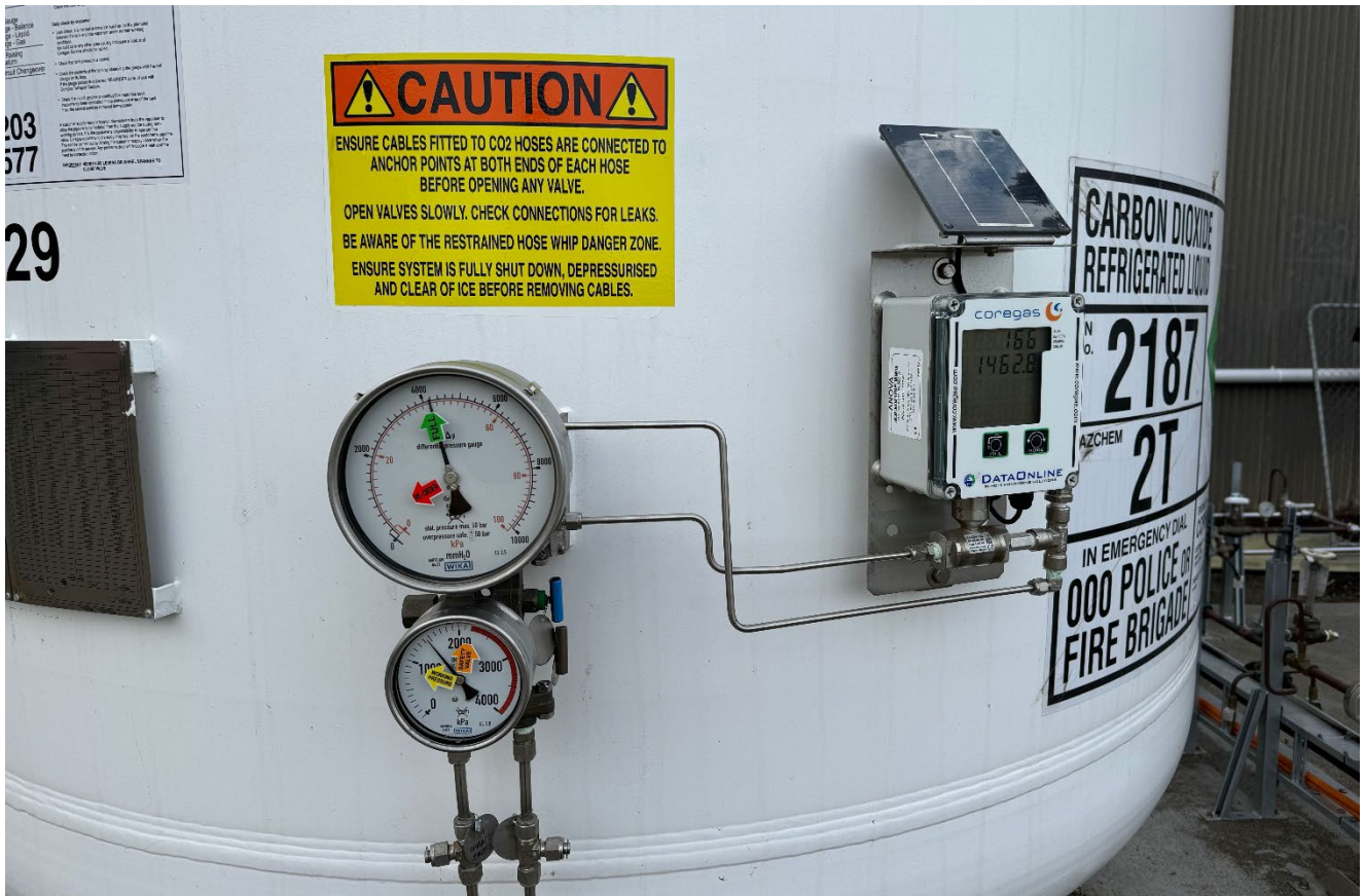
Figure: Coregas Oxygen and Carbon Dioxide tanks operational
