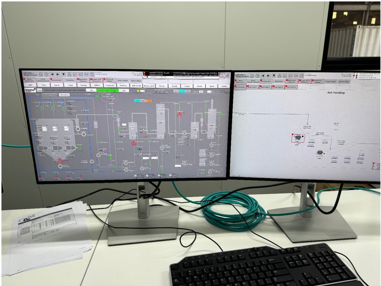
Figure: SCADA system commissioning ensuring signals to equipment is correctly received and controlled
