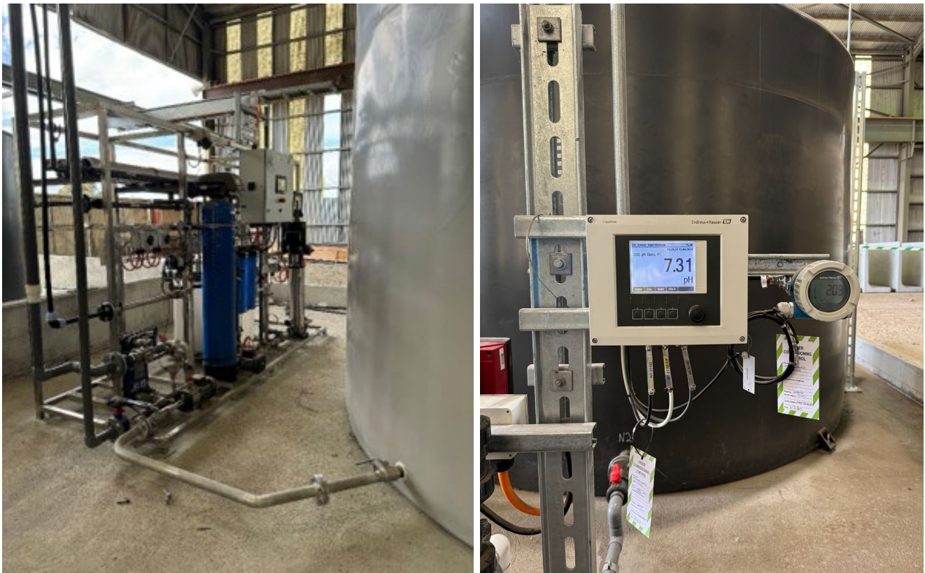
Figure: RO Plant and Raw Water equipment operational
