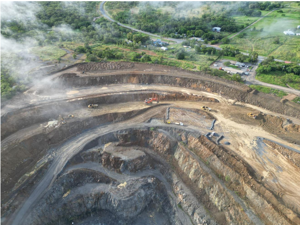
Picture above: Stripping ongoing with the noise and visual bund construction progression.
