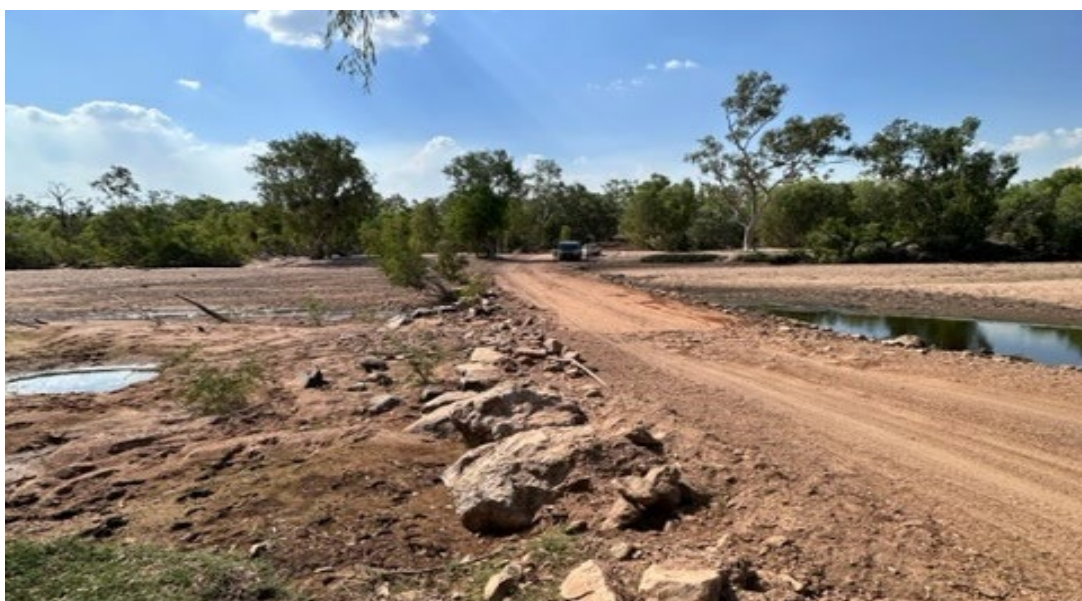
Robinson River crossing looking north on the Agate Creek-Forsayth road – 13 December 2023
