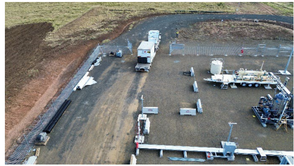
Figure 2: First cargo of HDNG leaves facility
