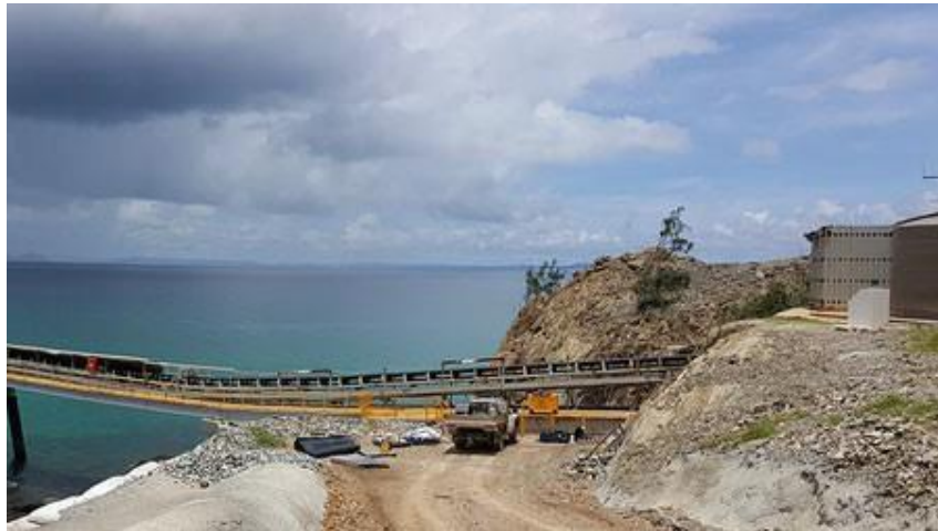
Figure 33: Lack of space on existing conveyor structure for a second conveyor.
