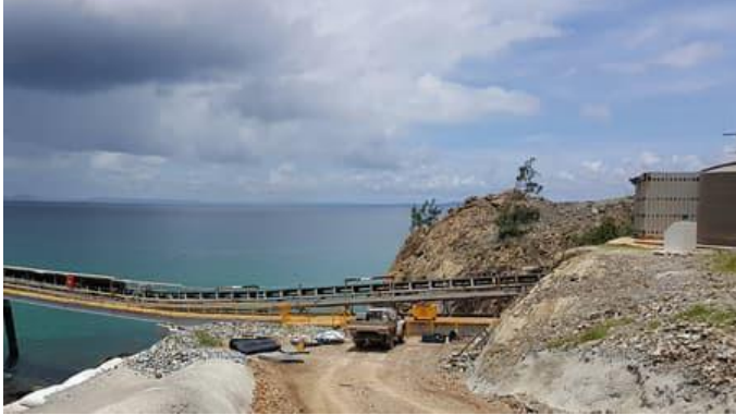
Figure 3233: Lack of space on existing conveyor structure for a second conveyor.
