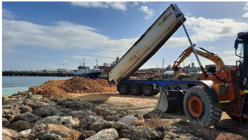
Figure 16: FEL, excavator and dump truck working to place fill for typical armoured rock wharf
