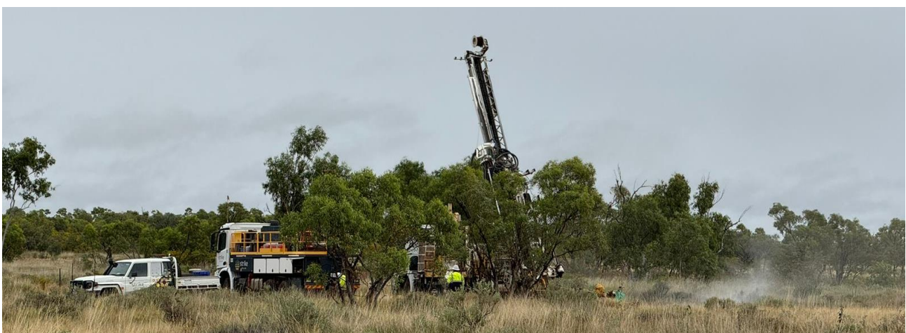
[Figure 1] Sybella Project: weathered, transitional and fresh REO-enriched granite (top). Note the coarse grain-size, weak biotite deformation fabric and increased fracture density with increased weathering. Step-out drilling in progress (bottom).
