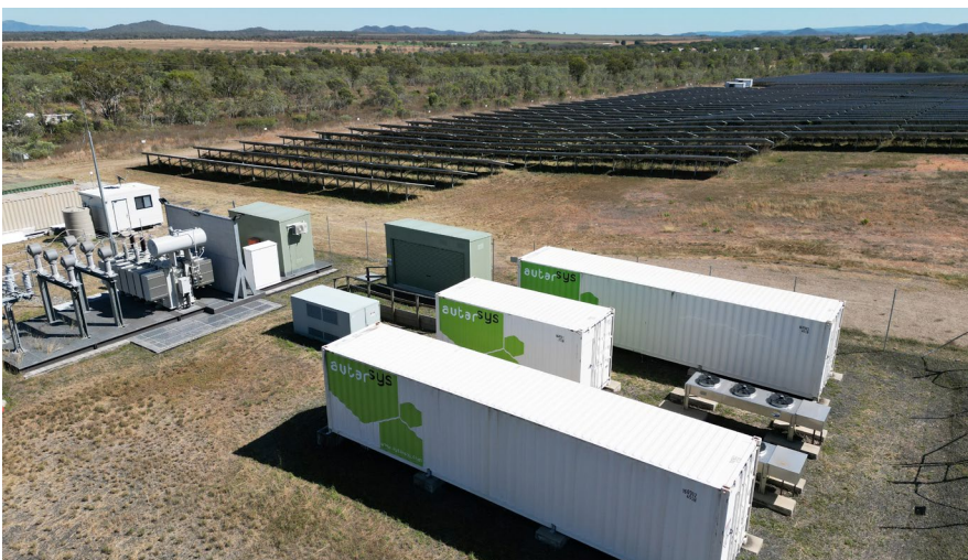
Image: Lakeland Solar & Storage Project (QLD)
