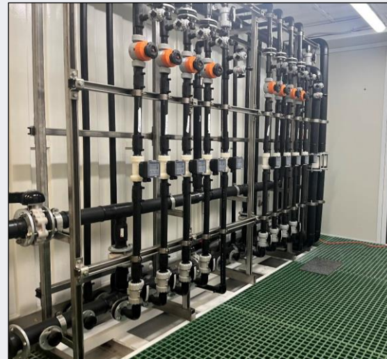
Wellhouse Module (pipe room)
