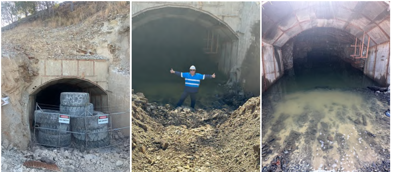
The existing portal to the 430m decline re-opened mid-July 2024, with Anthony Bainbridge, Chief Geologist, for scale.
