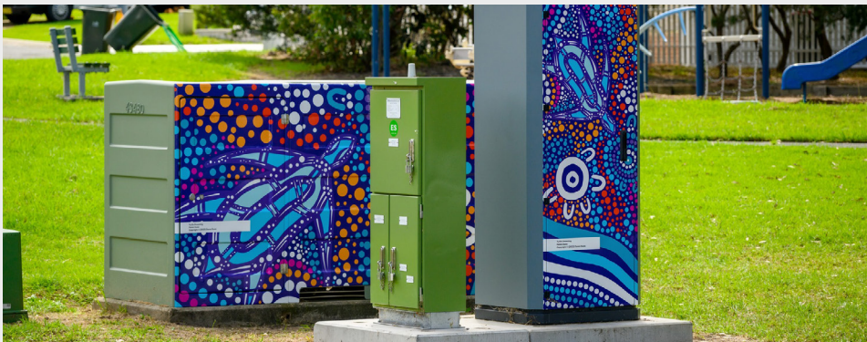
Community battery at Shell Cove, New South Wales.
