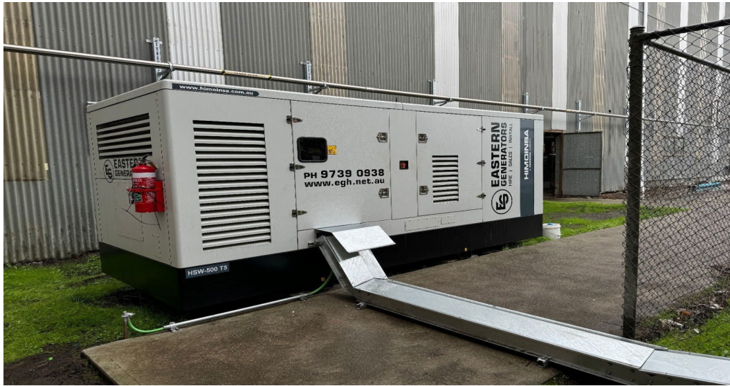
Emergency Standby Generator installed
