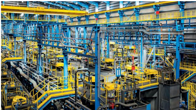
MATSA's brand new 4.6 Mt per year treatment plant
