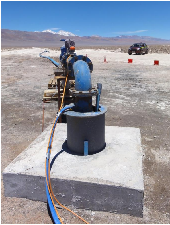
Figure 3: P4 pump and pipeline
