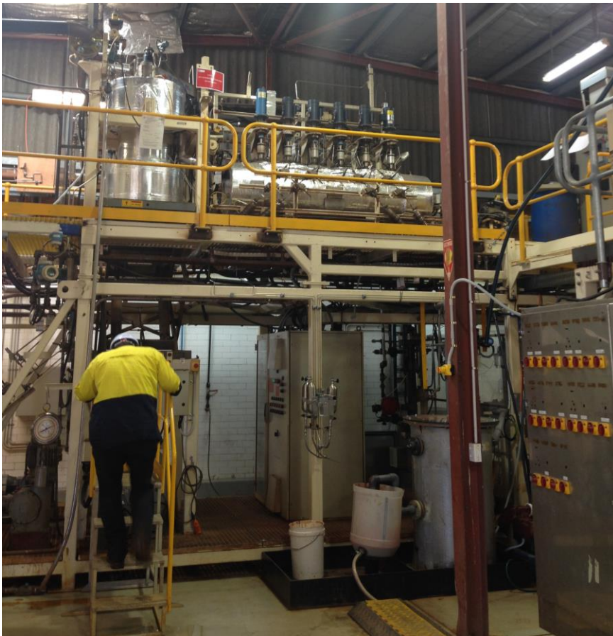
Figure 3: Pilot Plant: High Pressure Acid Leach Autoclave (horizontal cylinder at top of photo)
