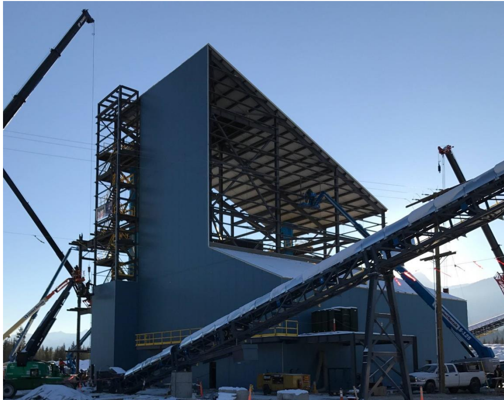
Load out conveyor and Process building
