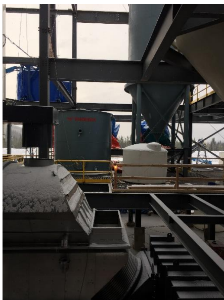
Equipment in Process building
