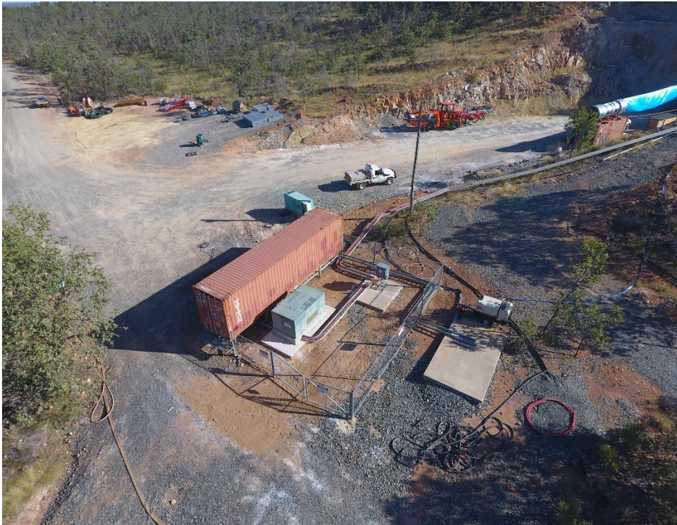
Figure 8 West 45 Portal Transformer
