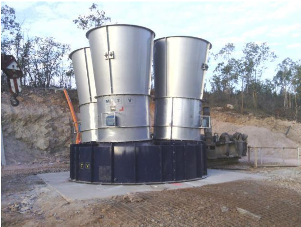
Figure 9 Ventilation fans installed at Return Air Raise (RAR)
