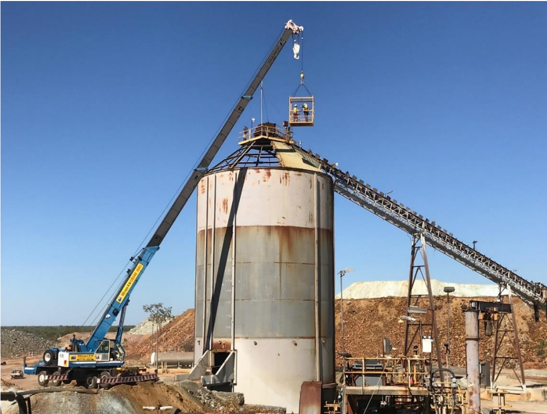
Figure 2 Roof sheeting being removed to inspect Fine Ore Bin top support structure
