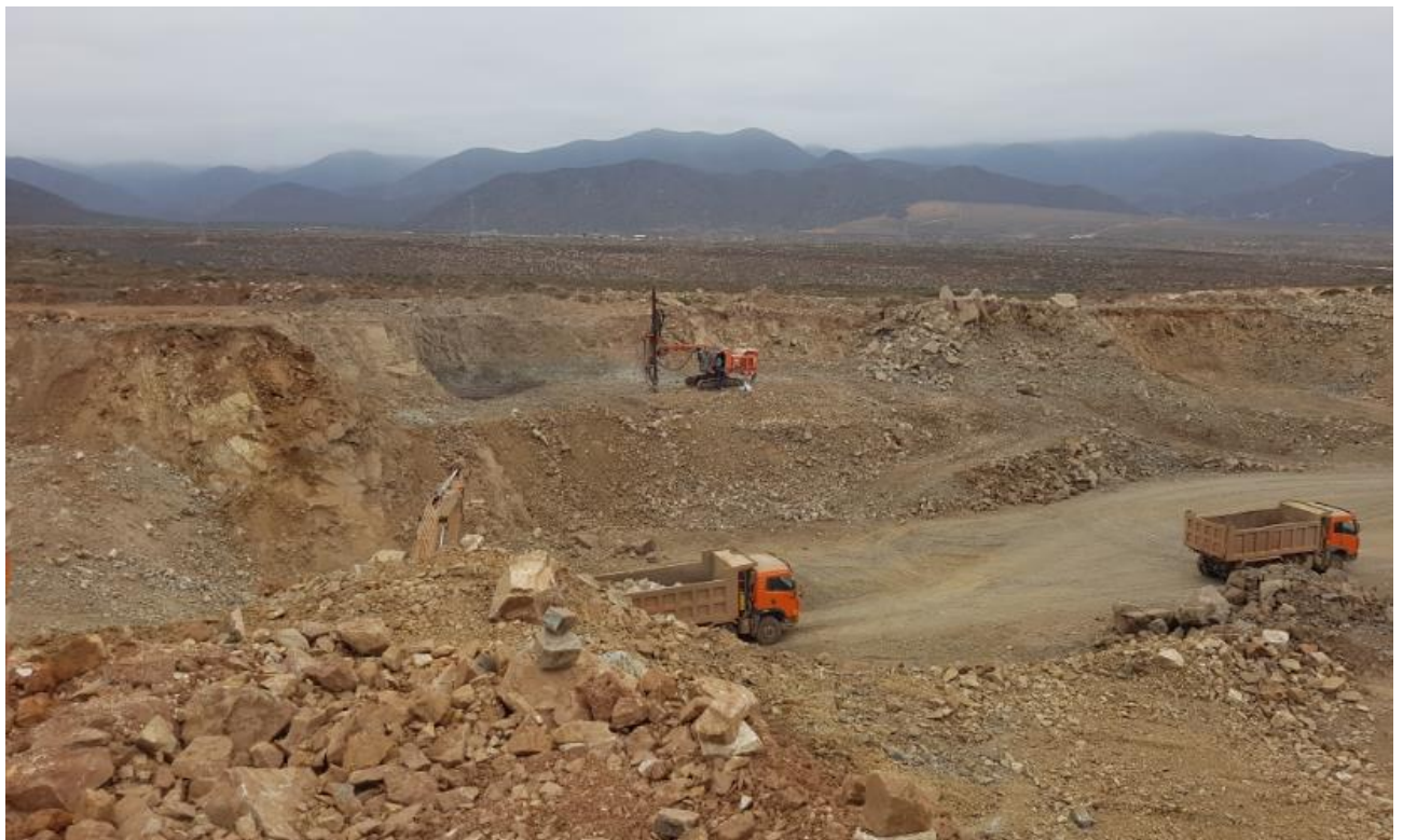
Figure 3 – Blasting drill rig preparing next bench for production blast. Trucks moving ore to demonstration crushing plant
