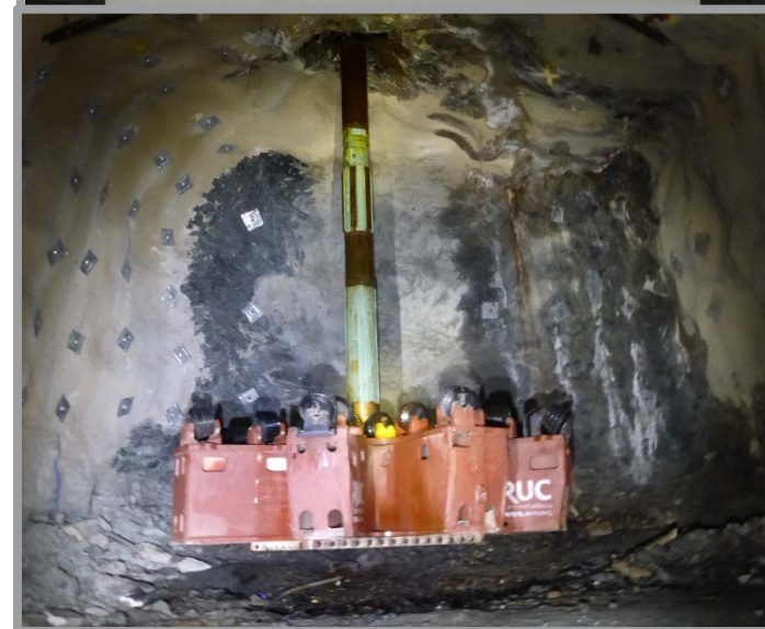
Above PAF equipment (mixer) on-site at Gwalia. Below: Reaming head of raise bore, January 2018
