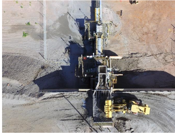
Primary crusher (overhead view)
