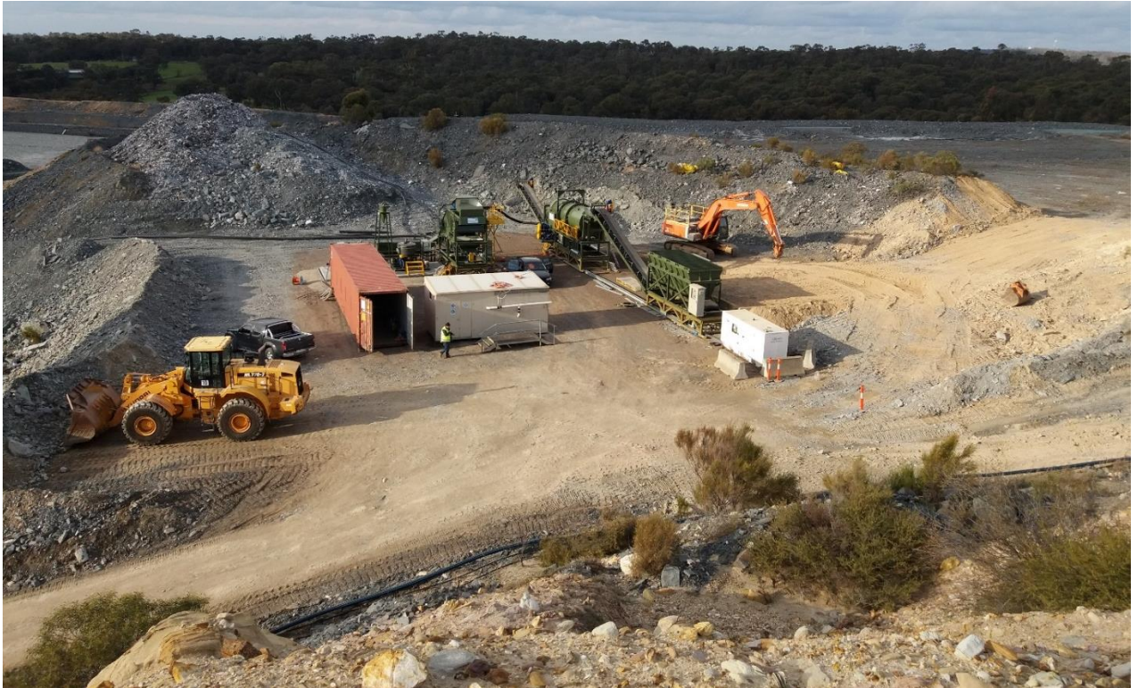
Figure 3: Kangaroo Flat Coarse Sand Dam Processing Equipment
