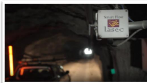
Readers connected through mine network to central control room
