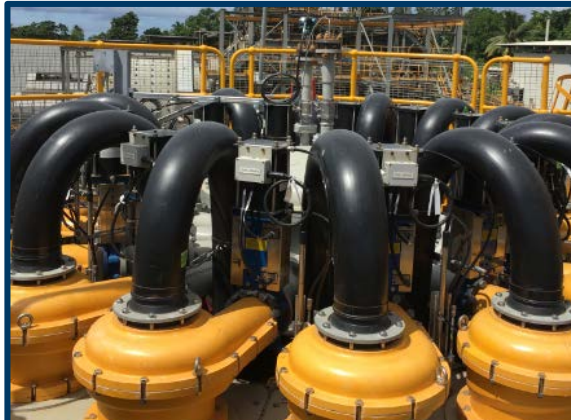
Float residue scavenging
