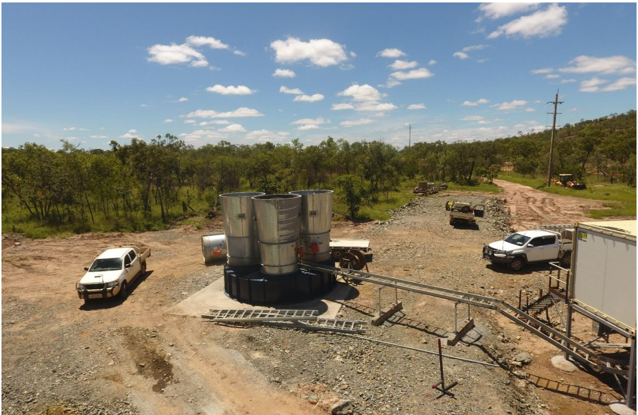
Figure 1 Far West Vent Fan Installation
