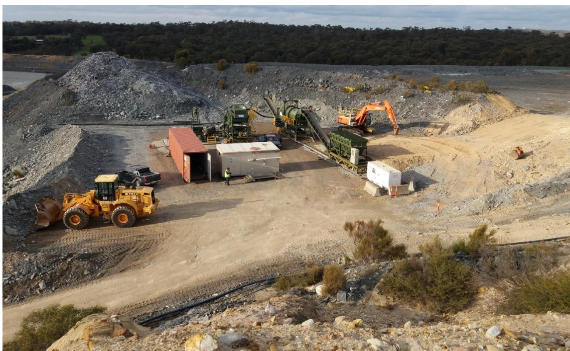
Figure 4: Kangaroo Flat Coarse Sand Dam Processing Equipment
